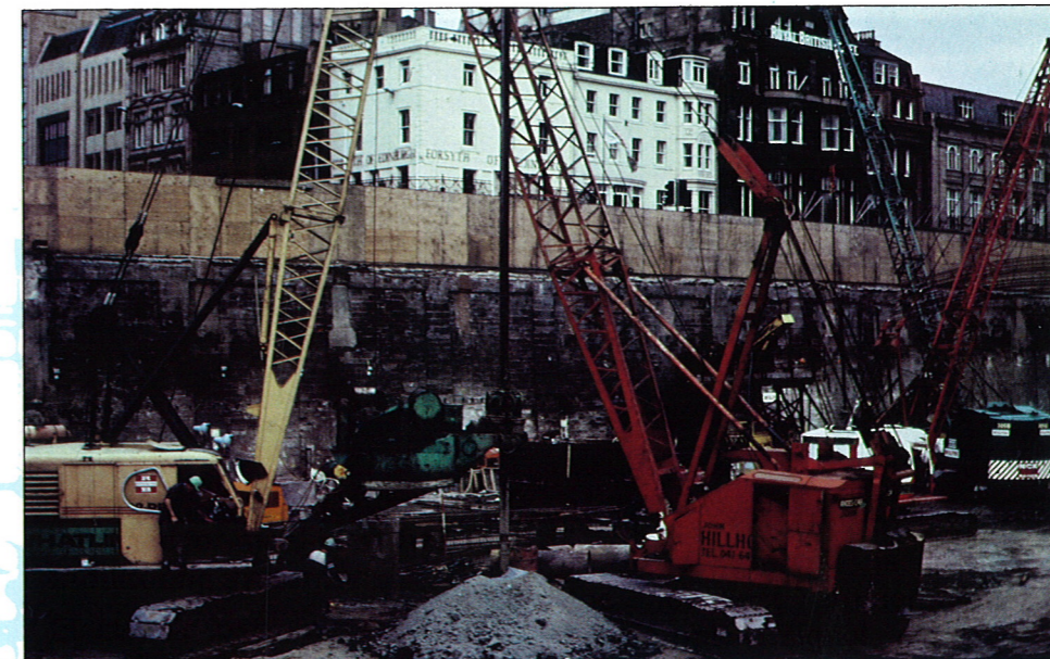
Early stages of Edinburgh Waverley Market Shopping Development showing old wall and Princes Street shops.
